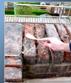
Removal of loose brick and cementitious pointing from the parapet coping stones
